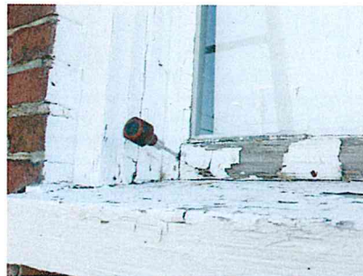
View of Failed Window Joint
