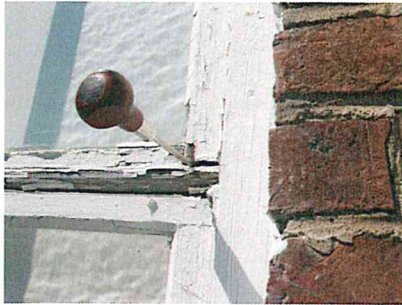
View of Failed Window Joint
