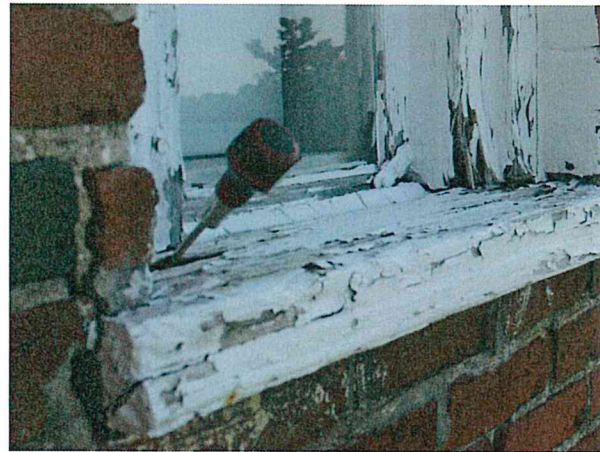
Close up View of Damaged Window to be replaced
