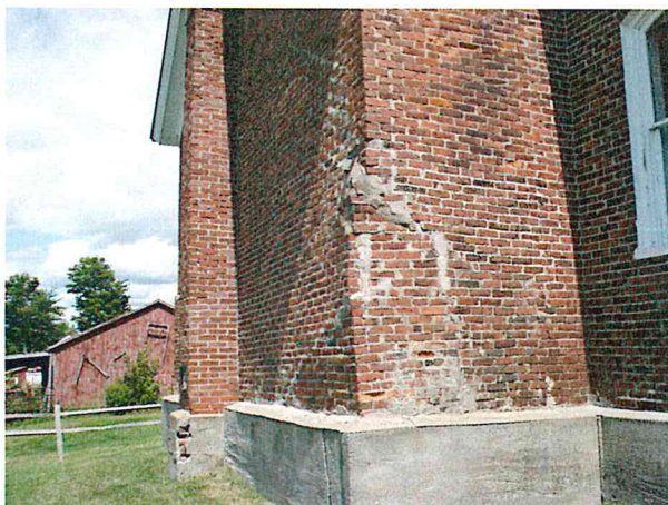
View of Brick Veneer in Poor Condition
