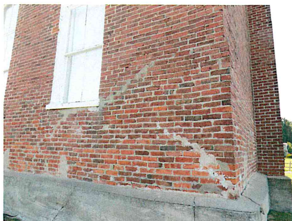
View of Brick Veneer in Poor Condition
