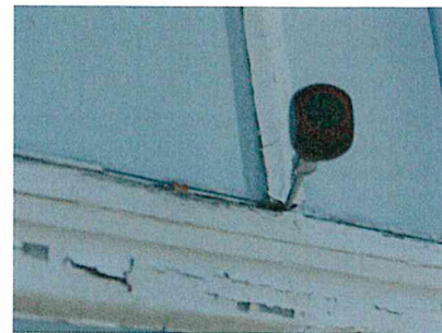
View of Failed Joint at Muntin Bar
